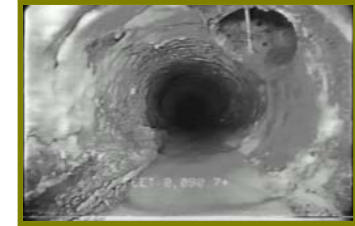
A sewer main coated with grease.
