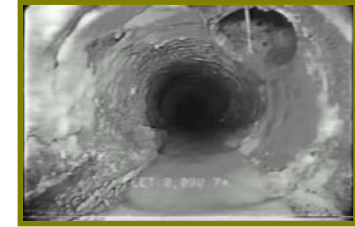
A sewer main coated with grease.
