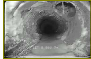
A sewer main coated with grease.
